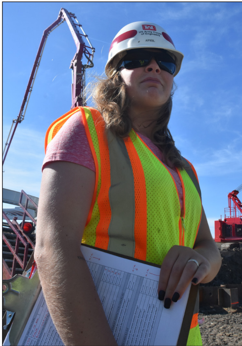
April McCann, construction representative, inspects the Fargo-Moorhead Metro Diversion Inlet structure, near Horace, North Dakota, Aug. 11. USACE photo by Patrick Moes
