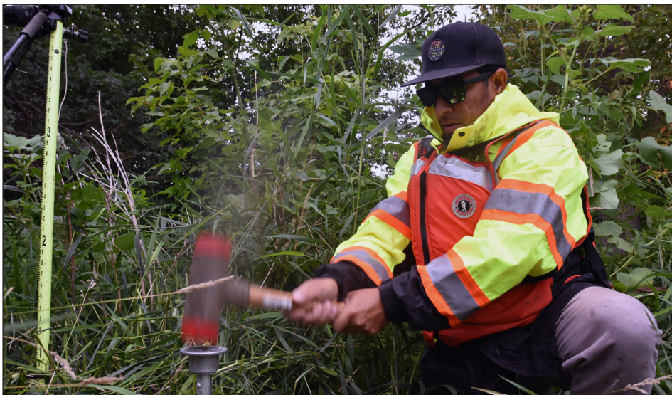
Eduardo Torrens, civil engineer, uses a hammer to drive a survey monument into the ground along the Red River of the North, near Georgetown, Minnesota, Aug. 12. USACE photo by Patrick Moes
