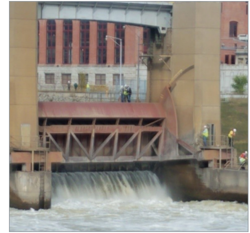
St. Paul District engineers perform safety checks of the Lower St. Anthony Falls Lock and Dam in Minneapolis, during a periodic inspection Oct. 6. USACE photo by Elizabeth Stoeckmann
