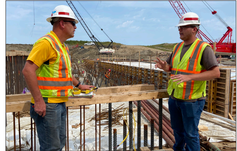
Duane Perkins, structural engineer, and Greg Hammons, construction representative, stand at the Fargo-Moorhead Metro Diversion Inlet structure, near Horace, North Dakota, Aug. 24. USACE courtesy photo
