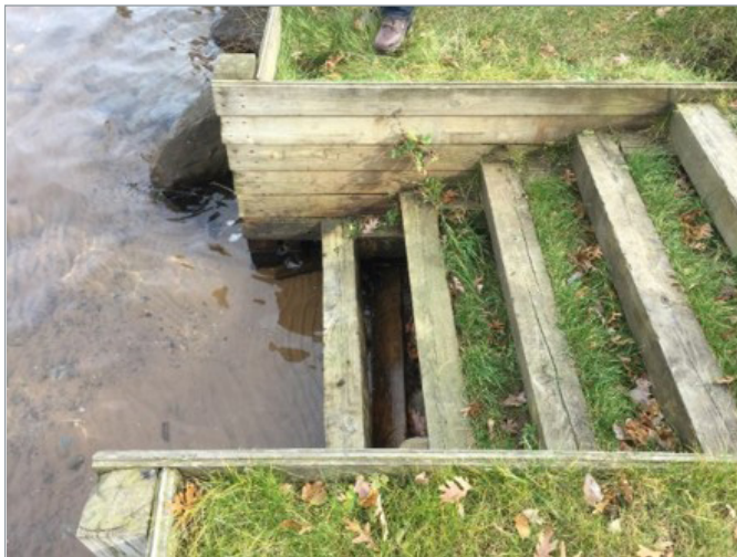
Erosional damage to tribal infrastructure, in south central Burnett County, Wisconsin. USACE courtesy photo
